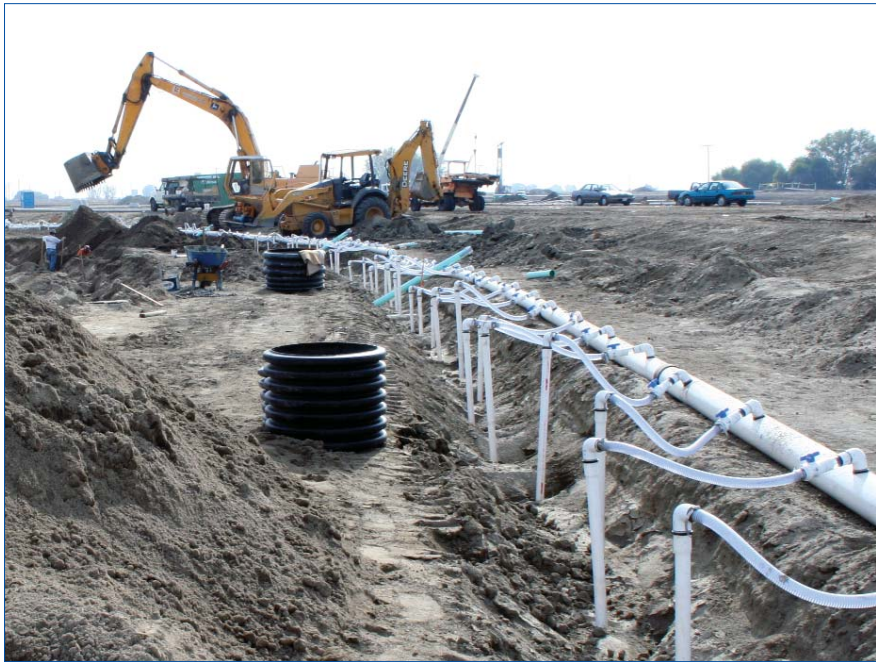
In a wellpoint dewatering system, a series of shallow wells is installed along the side of the excavation in which the pipe will be laid.
