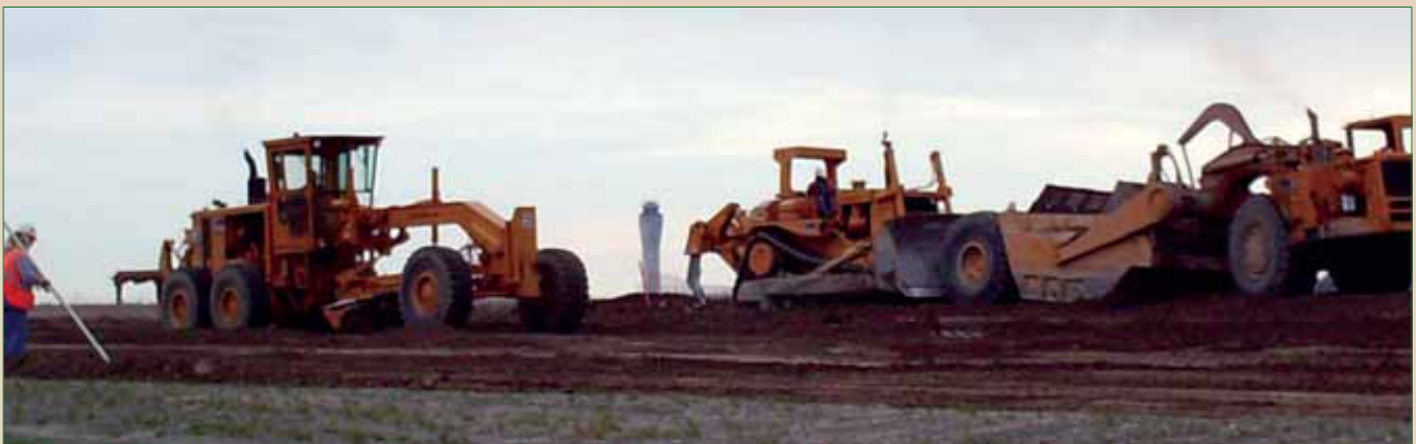
By performing both grading and utility work, SCI gives clients one less subcontractor to coordinate with. This also eliminates the question of who is responsible for compacting soil throughout the site.
