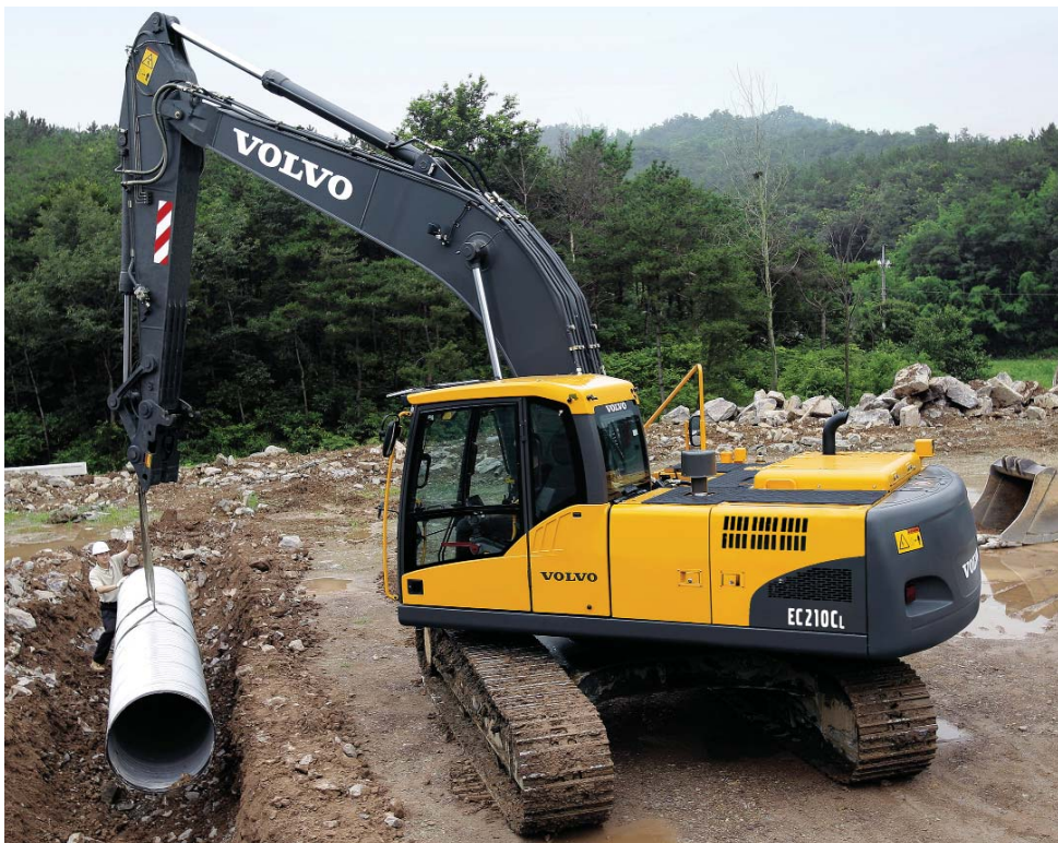
Attachments are an important factor for a utility contractor. Improvements in excavators' hydraulic systems have made a variety of attachments more efficient and easier to use.
