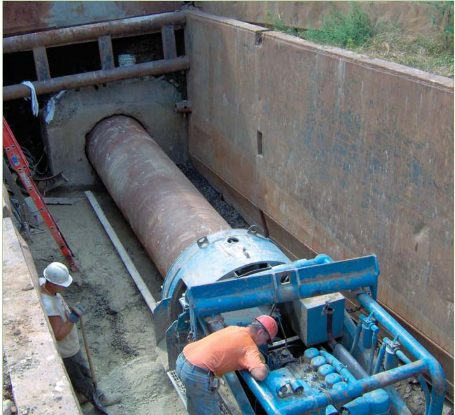
Planning is the key to making health and safety efforts work, according to Bill Santa, safety coordinator for Alex E. Paris Contracting. That means setting objectives, identifying hazards, assessing risks and implementing standards of performance.
