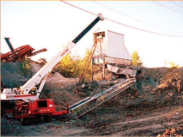
This NIOSH photo captures the aftermath of a fatal accident in which a crane boom made contact with an overhead power line.
