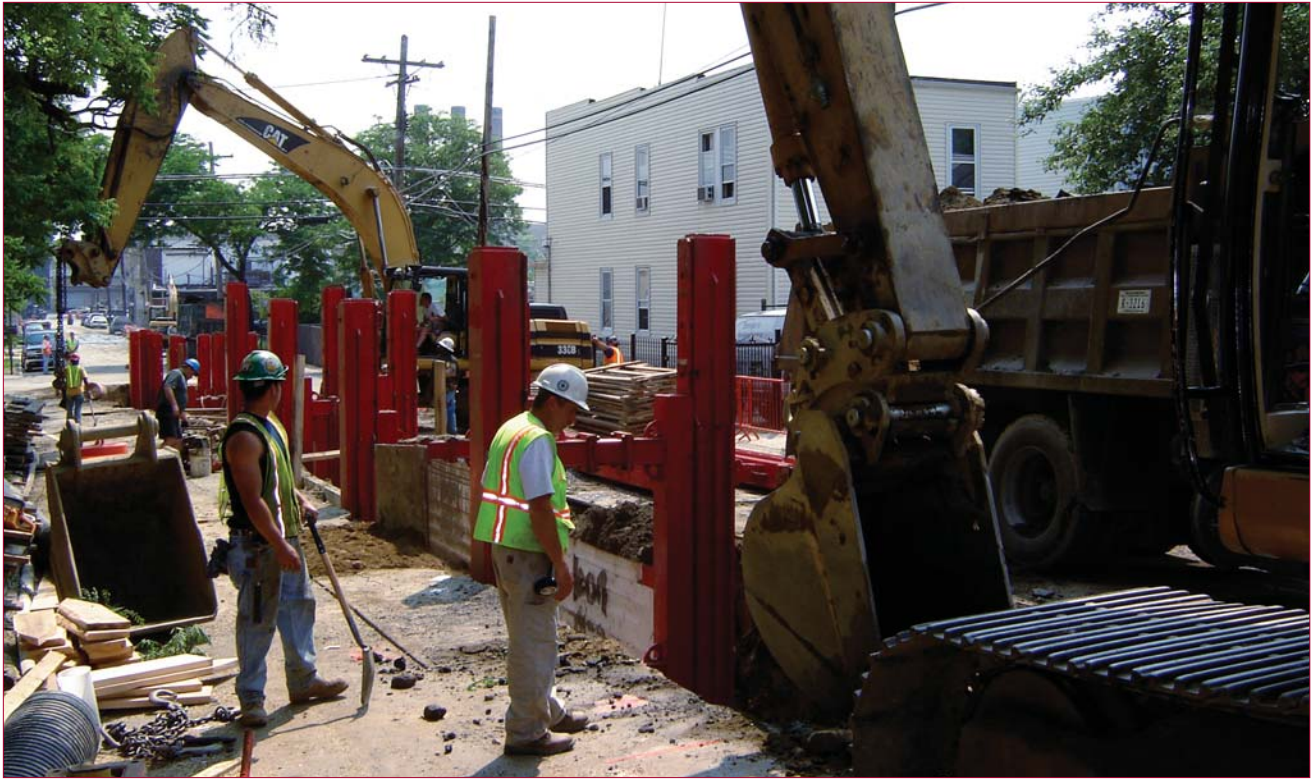
Early variations of trench shielding and shoring (at least as we know them today) began to take shape in the early 1900s using timber shoring, followed by steel boxes that were built by contractors as far back as the 1930s.
