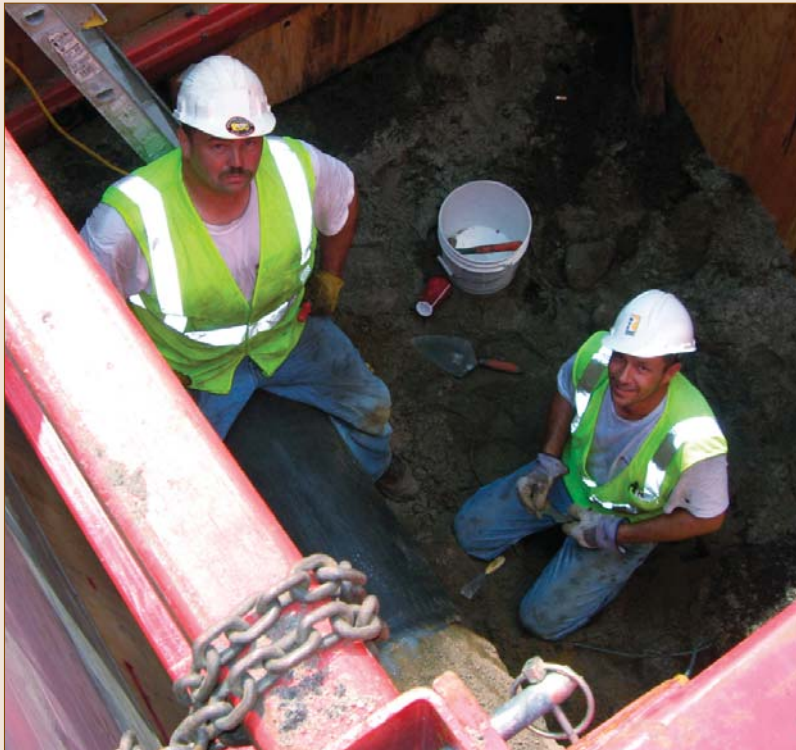
Harold Enberg and Dan Miller of Minnesota Utilities & Excavating on the job at Hope Lodge.
